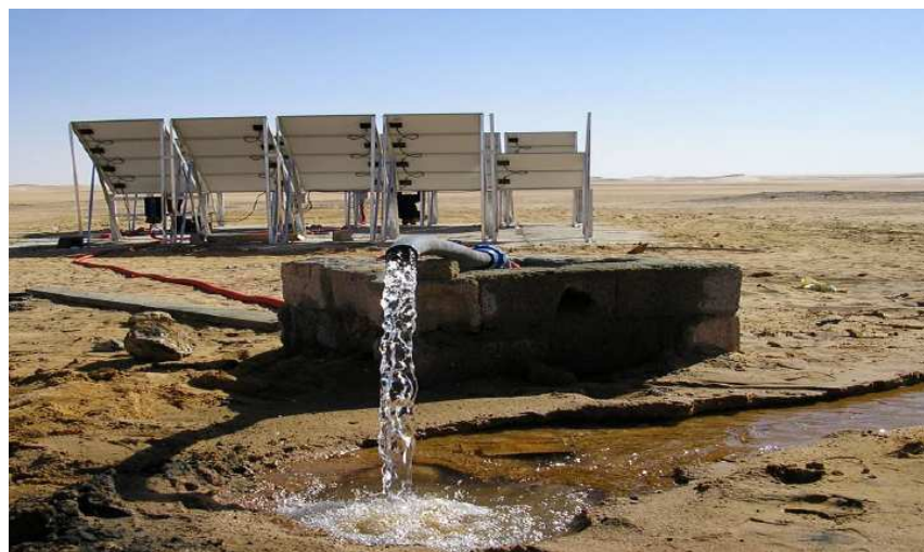
Figure 2-15: PV Water pumping for livestock
