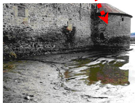
Figure 5 – Piping system in moat
