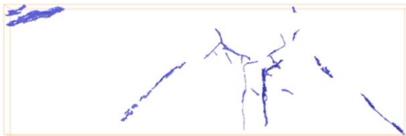
Fig. 2. Crack structure by planar tomographic investigation
