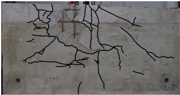
Fig. 1. Crack structure of the underside of S26P02
