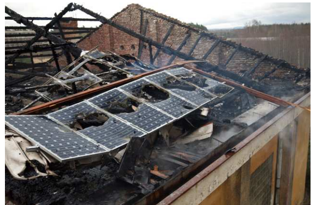
Fig. 1. Roof mounted PV power plant after fire.
