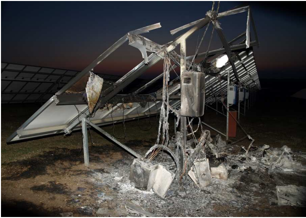
Fig. 2. Stand alone PV power plant after fire.
