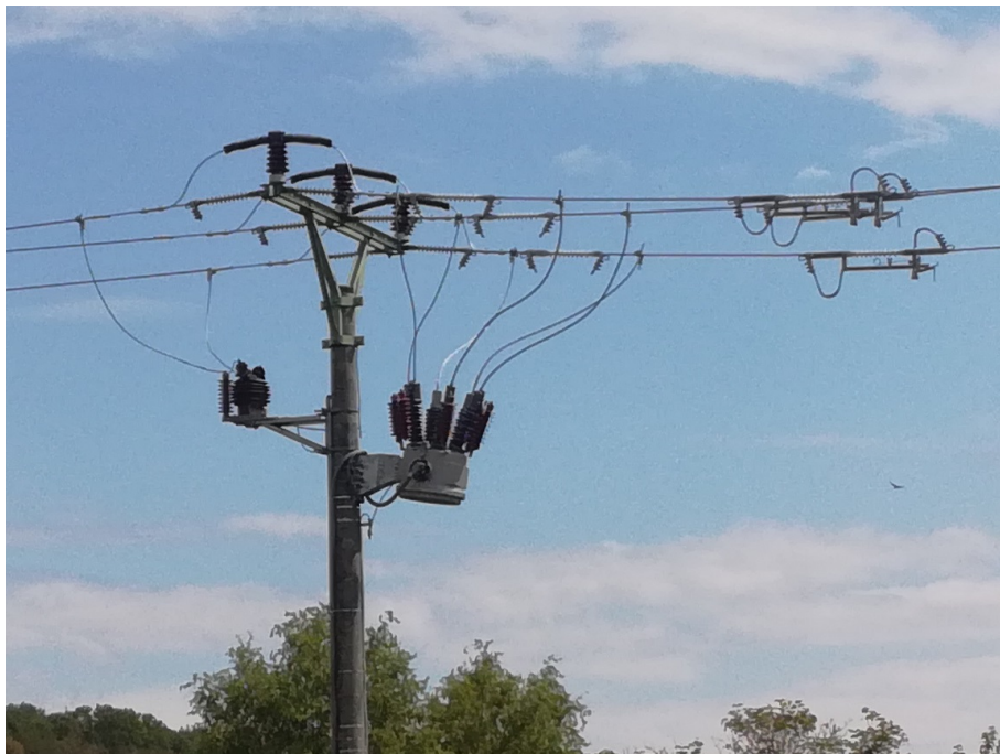
Obr. A.7: Recloser v provozu
