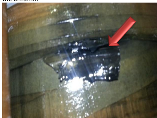
Fig. 6: Detail of the insulation of the HV coil of the transformer
