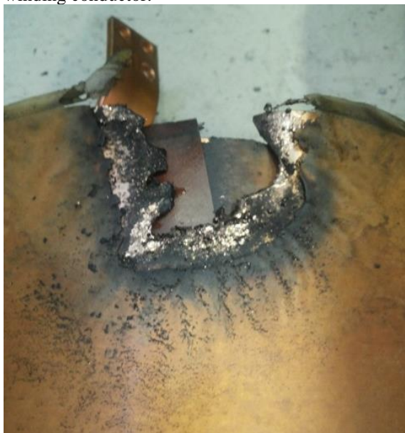
Fig. 12: Detail of the molten winding of the LV transformer coil.
