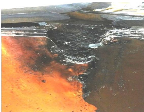
Fig. 11: Combustion site at the point of short circuit, where an electric arc has formed, which has led to deterioration of the insulation and melting of the winding conductor.
