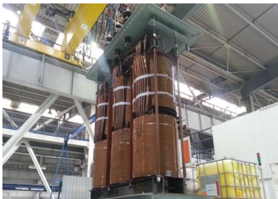
Fig. 4: Transformer pulled out of the oil vessel. The electrical insulation system of the transformer consists of combined dielectrics: mineral oil and paper.
