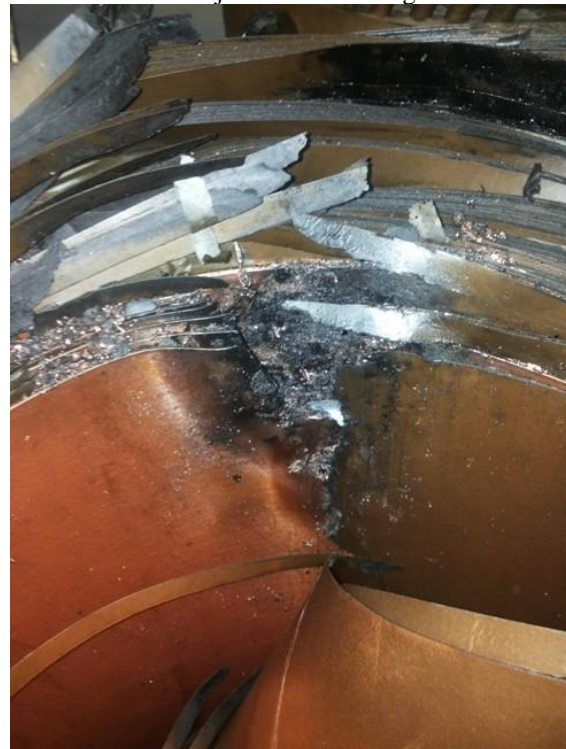
Fig. 10: Detail of the location of the interturn short circuit on the LV coil of the transformer. The interturn short went through 9 layers of the winding.
