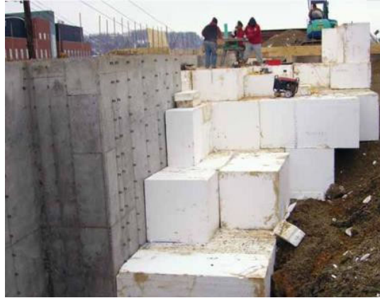
Figure 1-11: West Virginia University student housing project (Morgantown, West Virginia) with EPS geofoam retaining wall backfill [4]
