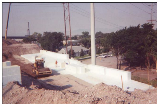
Figure 1-5: Construction of 100 South Street and I-15 with EPS geofoam. Note the proximity of operations with houses and power lines [9]
