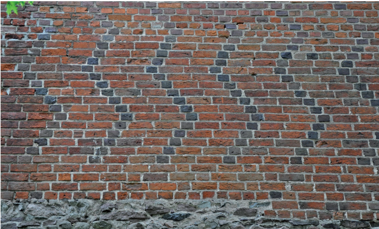
Fig. 16. Bierzłowo (Bierzłowo castle). Pattern of burr brick on northern façade of northern circumferential wall. Photo B. Wasik.
