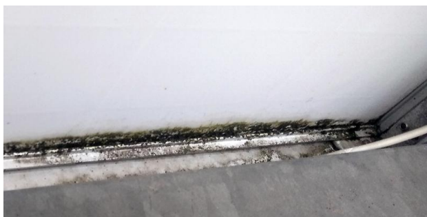
Fig. 7. Panel backside - biological corrosion (Pilsen, CR, 2021).
