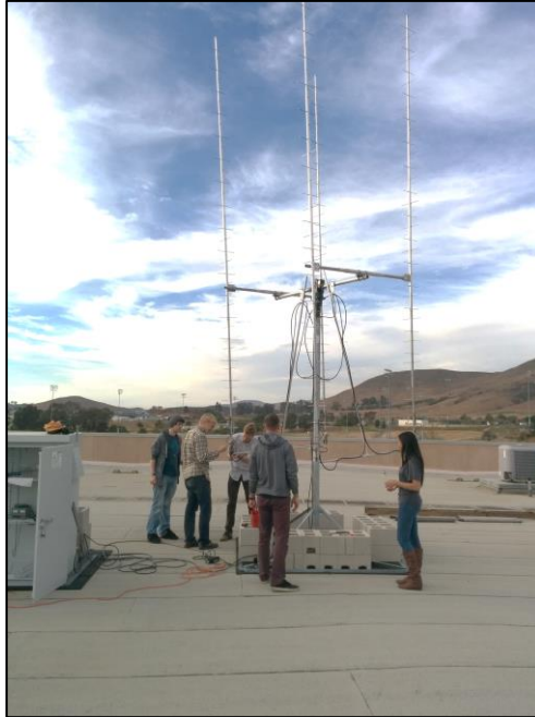
Figure 11. An installation picture of the new Cal Poly's GS named "Friss" with four phased Yagi antenna to track LEO satellites at 437 MHz [17].
